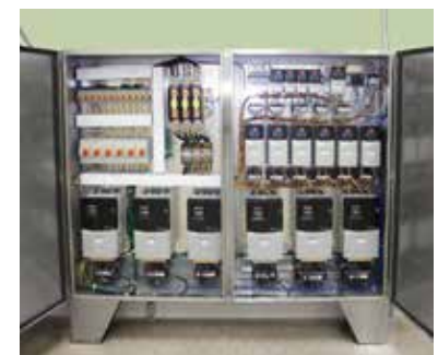
Control Panels & Devices
